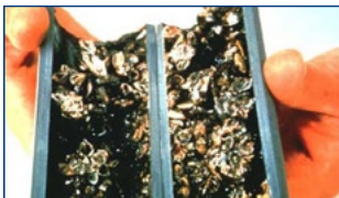
Water intake pipe blocked by zebra mussels
